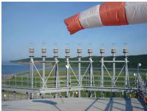
Figure 10 Example of LNG Tank Pressure Relief Valve
