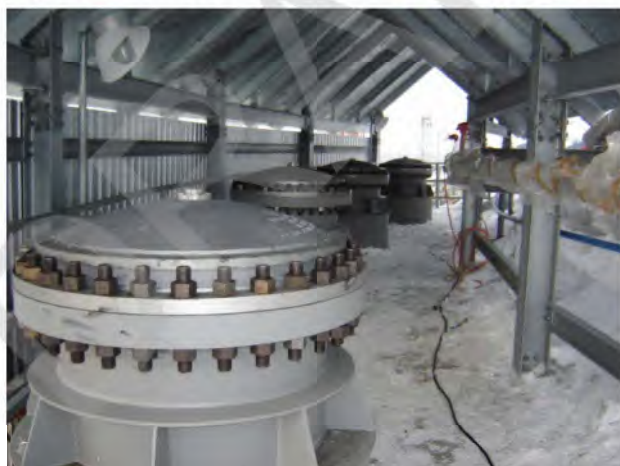
Figure 11 Example of LNG Tank Reserve Capacity Valve
