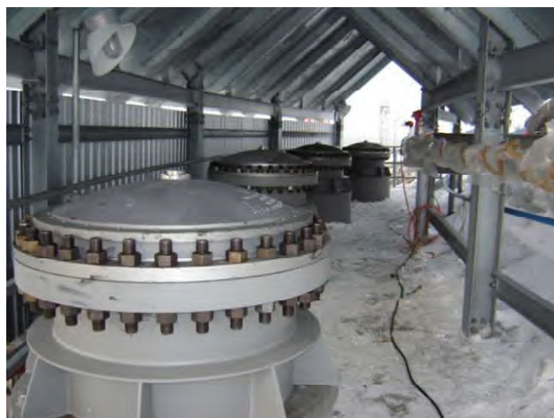
Figure 11 Example of LNG Tank Reserve Capacity Valve
