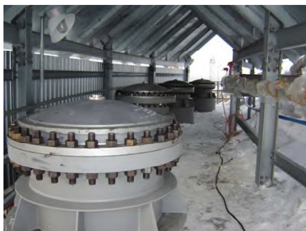
Figure 11 Example of LNG Tank Reserve Capacity Valve
